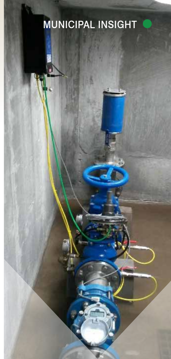
Typical pressure reducing valve installation in Overstrand
